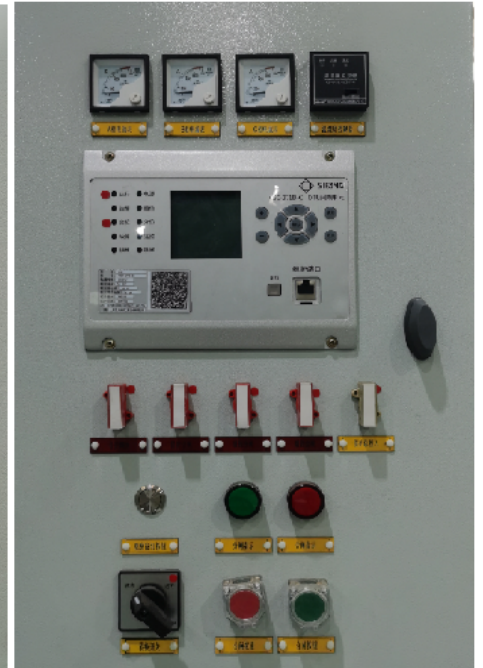
Remote and local control
